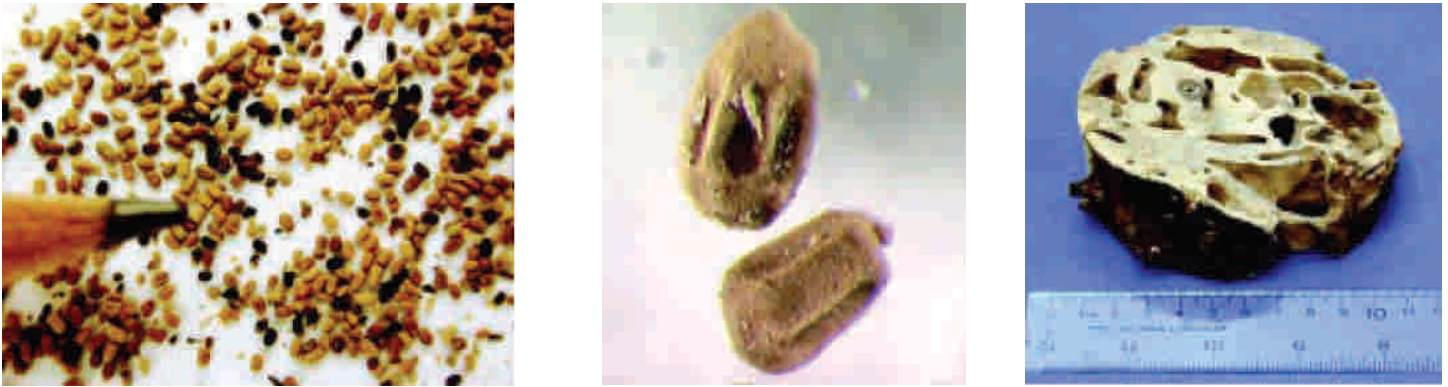
Figure 3. Drywood fecal pellets and damage
